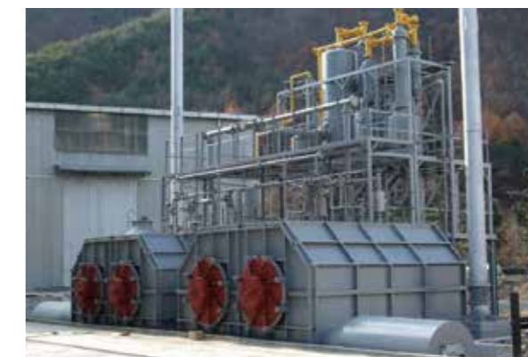
▲ Waste plastics liquefaction equipment
